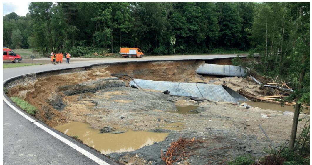
Picture 5: Damage due to a blocked culvert in Bavaria.
