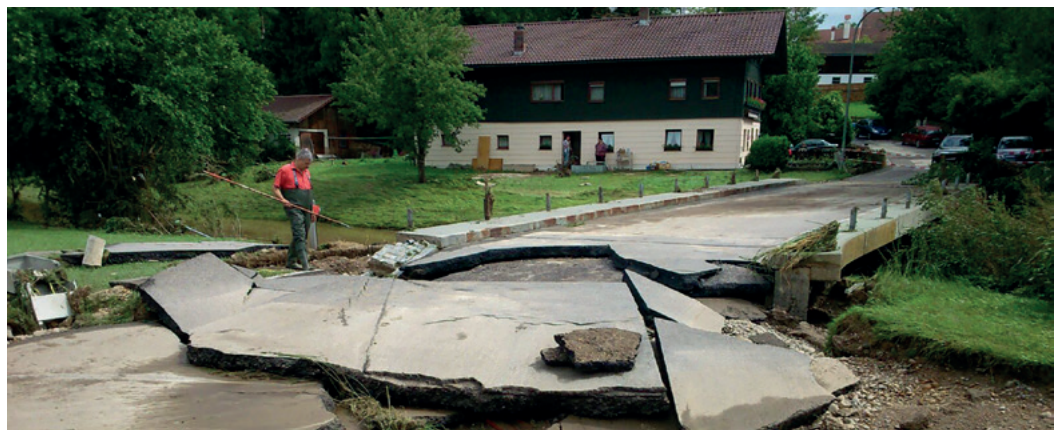
Picture 1: Destroyed road due to a creek flooding in Triftern, Bavaria.
