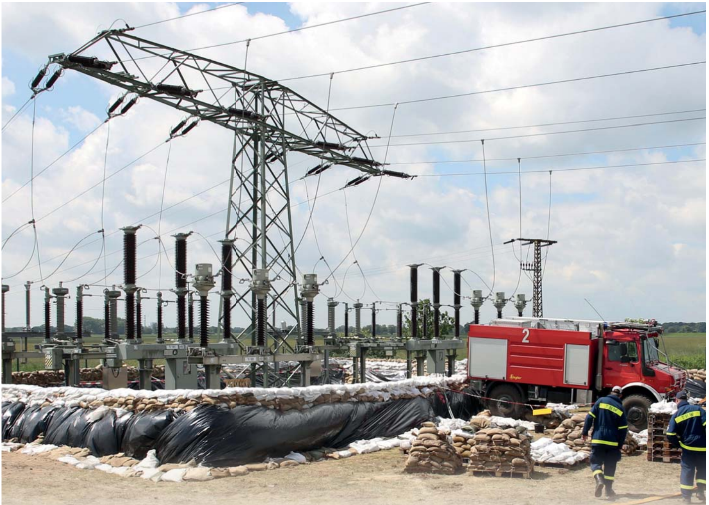
Flood damage near Stendal, Germany
