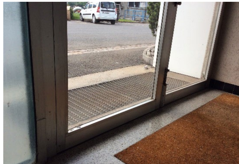
Figure 5: Doors and glazing should be impact-resistant and water-tight. Mobile flood protection may need to be considered for operations-critical areas.
