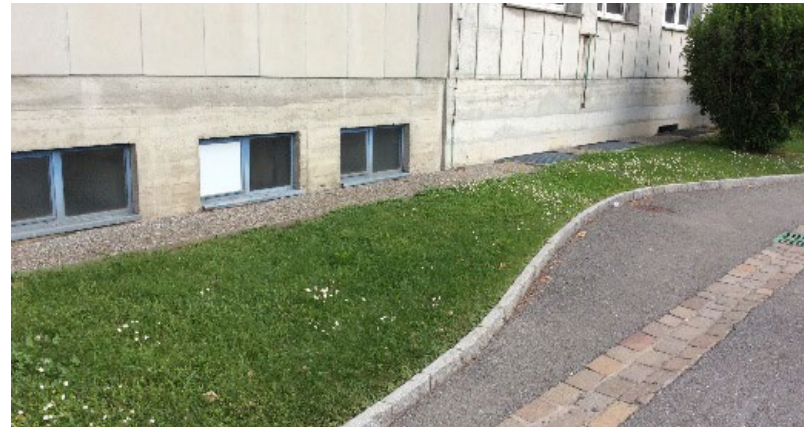
Figure 4: Openings on the ground floor should be above "design level" flood and provided with impact-resistant glazing or doors against water-borne debris. Mobile flood protection may need to be considered for operations-critical areas.
